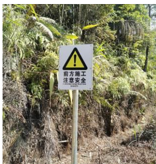
On-site warning signs
